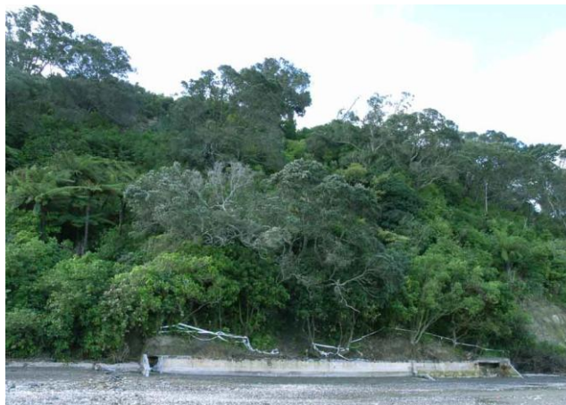
Fig. 3. Newly-demolished New Lynn Outfall ("Septic Tank" of Fig. 2). Forest above of pohutukawa, kohekohe and puriri. Photo: R Gardner, 15 Oct 2012.
